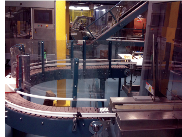
PACKAGING CONVEYING SYSTEM FOR ENERGY BAR MANUFACTURER, NBTY IN LONG ISLAND, NEW YORK
